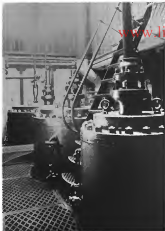
UPPER GRATING, ENGINE ROOM PRINCESS ANNE.
