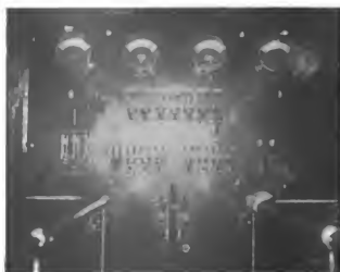
GENERAL VIEW OF SWITCH BOARD.
