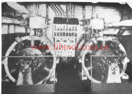
DIRECT CONNECTED GENERATING SETS, S.S. BREMEN.
