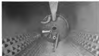
STEAM CHAMBER IN YARROW BOILER AFTER MISHAP.
