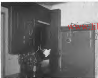
TELEPHONE EXCHANGE ON MAIN DECK.
