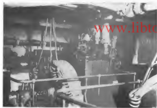
STARBOARD SIDE OF DYNAMO ROOM.
