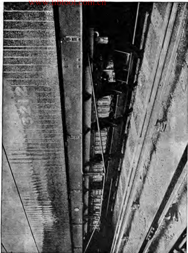
Fig. 377. Arrangement of Control Apparatus Under Car.
