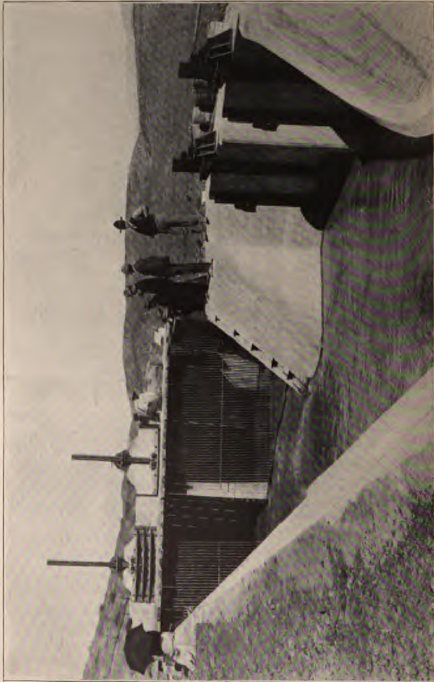
SLUICE GATES AND ENTRANCE END OF COTTONWOOD PRESSURE PIPE Salt River Project, Arizona.
