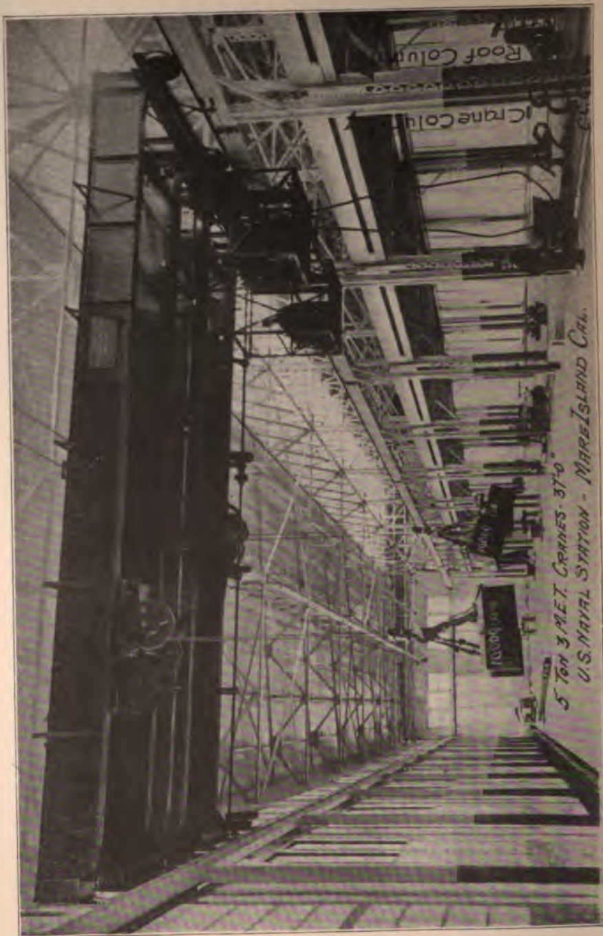
Fig. 117. Five-Ton Electric Travelling Cranes Installed at U. S. Naval Station, Marie Island, California. Courtesy of Cleveland Crane & Car Company, Cleveland, Ohio.
