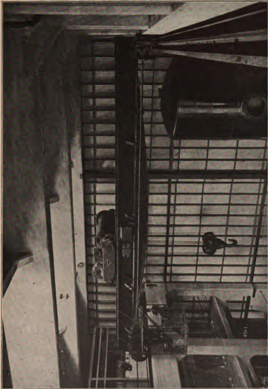
Fig. 107. Fifty-Ton Three-Motor Electric Traveling Crane. Courtesy of Northern Engineering Works, Detroit, Mich.
