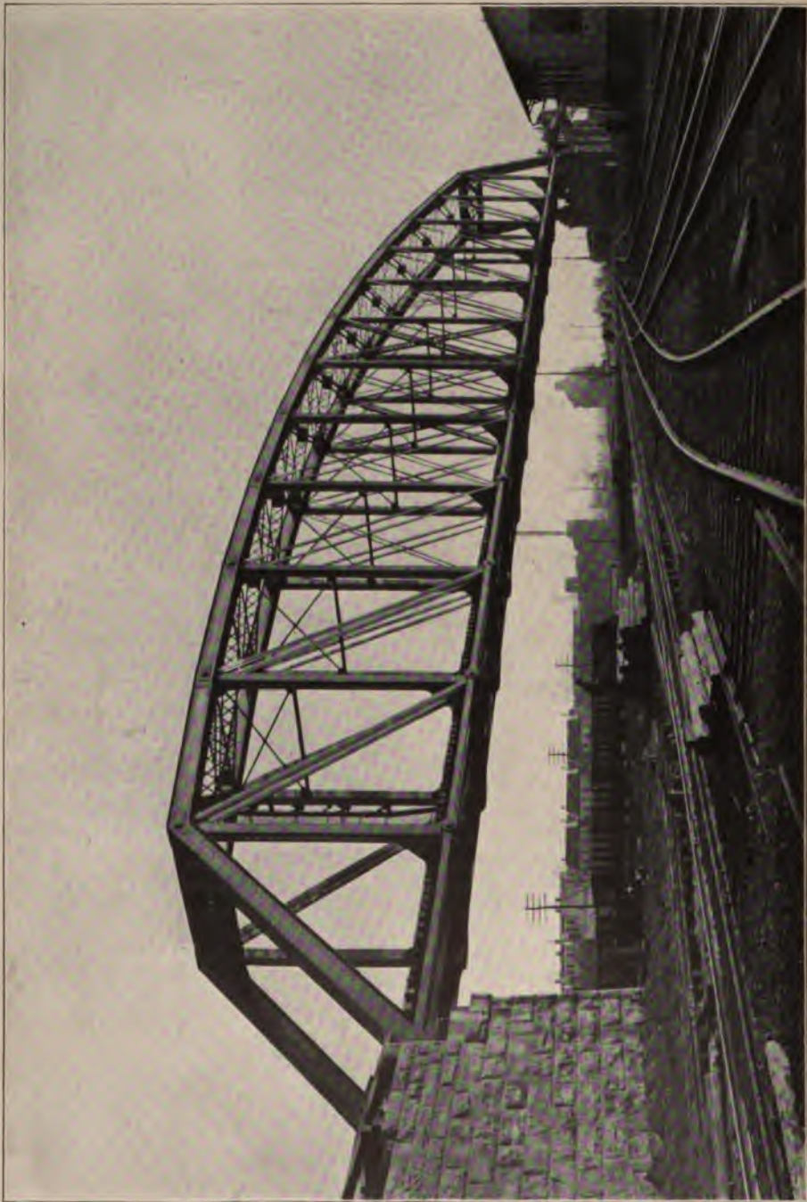
BRIDGE AT 52D STREET OVER FREIGHT YARD OF THE PENNSYLVANIA RAILROAD, PITTSBURG, PA.
