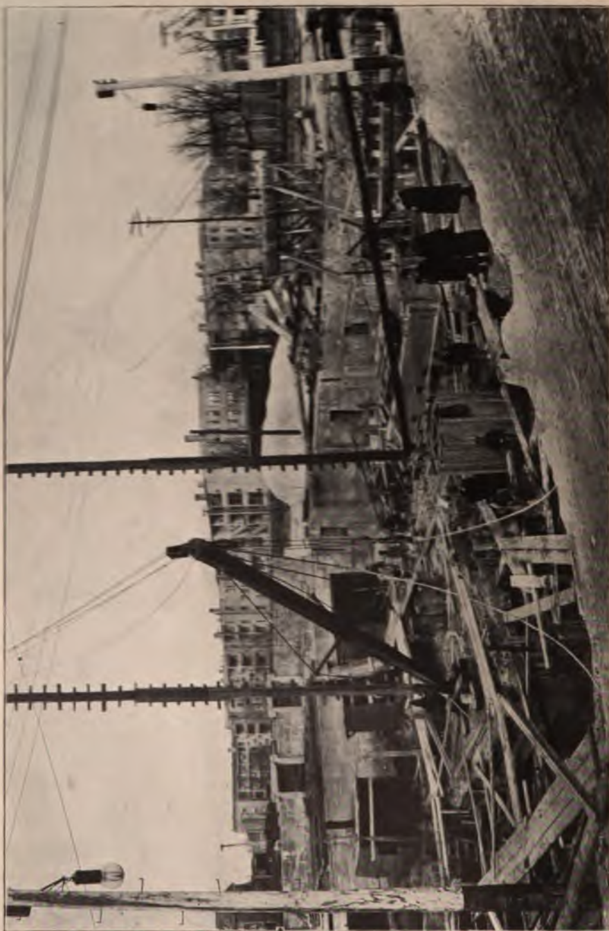
LAWRENCE AVENUE PUMPING STATION, SYSTEM OF INTERCEPTING SEWERS, CHICAGO, ILL., UNDER CONSTRUCTION
