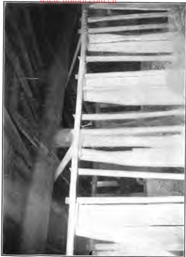
A TYPICAL BAD CEILING.
