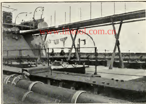
Pipe Lines, Deck Steam-pipes, Tank-tops with Guard Rails, and Fore-and-aft Bridge on modern Tanker. Note davit for supporting oil hose.
