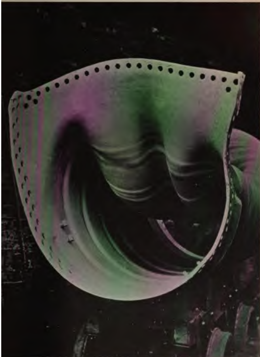
OVERHEATED BOILER FURNACE.
