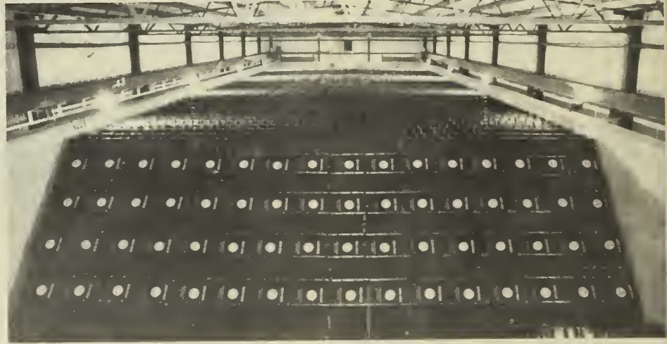
More than 19,000 drums of solidified radioactive waste are stored in this West Valley building.
