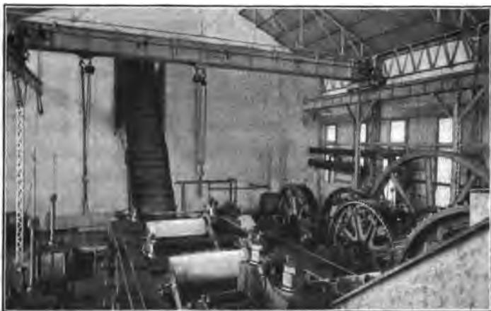
Interior of a crushing mill.
