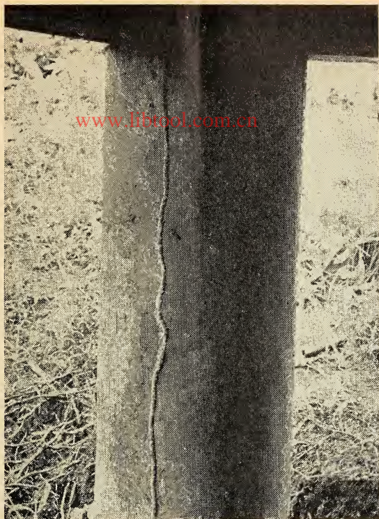
FIGURE 1.—Earthlike shelter tube constructed by subterranean termites over a heavily creosoted pine support of the test building (fig. 4) on Barro Colorado Island, Canal Zone.
