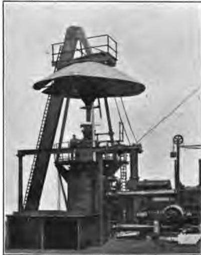
FIG. 35.—Power Gas Producer at London Paper Mill Co.'s Works. 1
