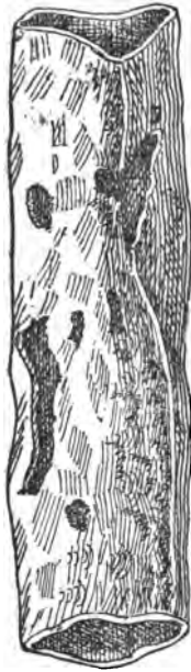
FIG. 19.—Lead Soil Pipe, unventilated and corroded by sewer gas.
